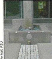
Infiltration of Roof Run-off
