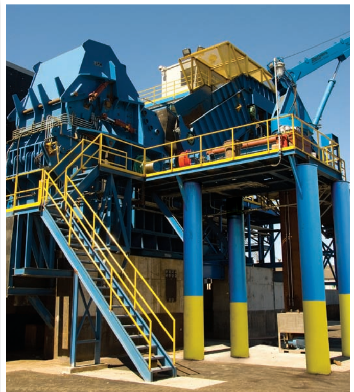
Schnitzer Steel's many investments at its Portland yard include a new mega-shredder. These improvements significantly enhance the operation's processing capabilities and global competitiveness.
