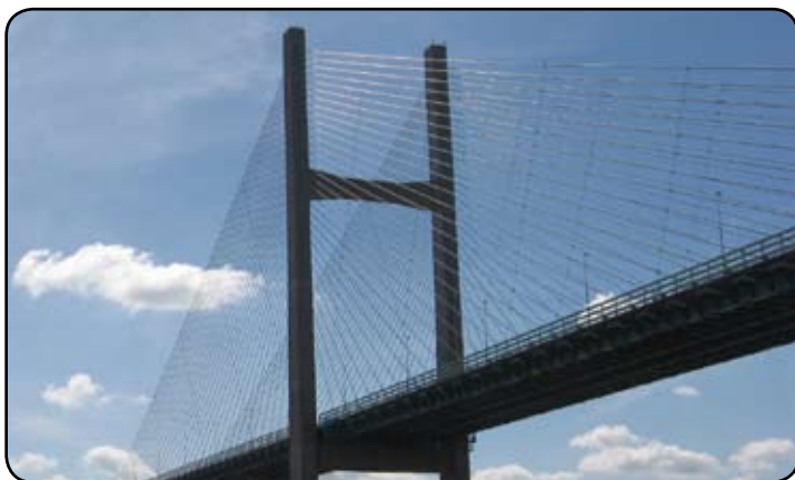
Second Severn Crossing between England and Wales in the United Kingdom. Image used under a Creative Commons license. Source: commons.wikimedia.org/wiki/File:Second_Severn_crossing.jpg
