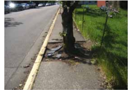
Sidewalk interrupted near Clackamas Regional Center.
