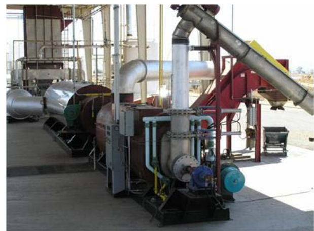
IES Pyrolysis Plant, Romoland, CA.
