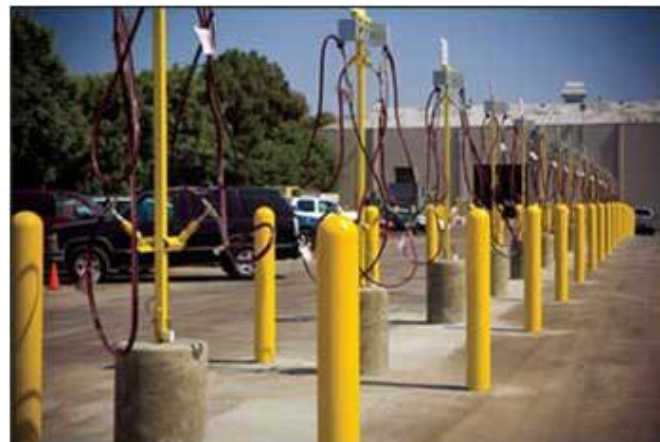
CNG Station, Fort Myers Beach, FL.
