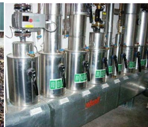
Combined heat-power manifold
