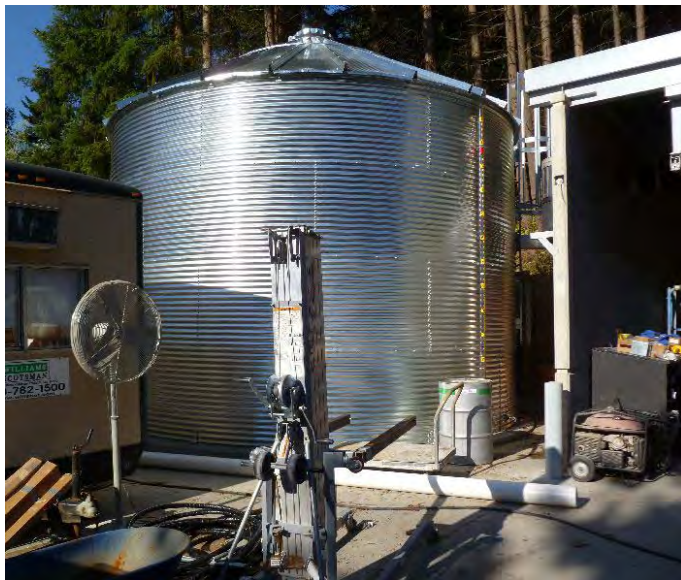
A 30,150 gallon tank captures rainwater from the Oregon Zoo's new Veterinary Medical Center.
