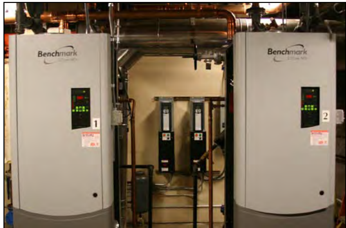
New energy efficient boilers at the PCPA Keller Auditorium are expected to save $10,000 annually in operating costs.
