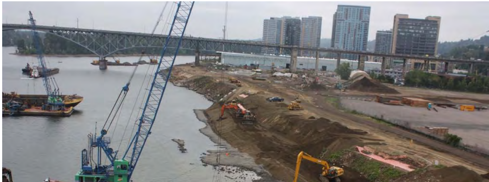
Portland South Waterfront. On-going cleanup of the Zidell property in foreground with high rise buildings in the background captures the phases of transformation of this area from historically industrial land to a modern mixed use waterfront.
