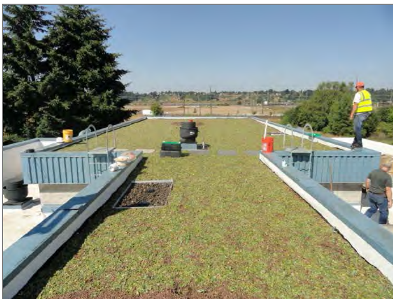
A 2,665 square foot ecoroof was added to the Metro Central Household Hazardous Waste facility in Northwest Portland.
