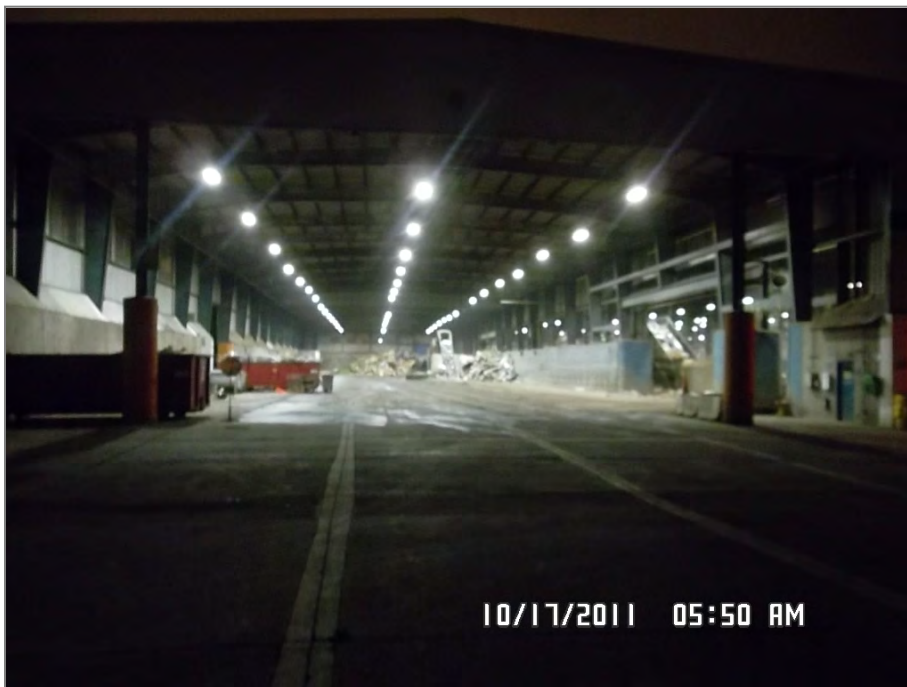
Upgraded lighting at Metro Central Transfer Station will use 28 percent less energy and provide better light for workers, especially during early morning shifts.
