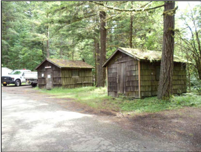
Degraded storage facilities Oxbow Regional Park
