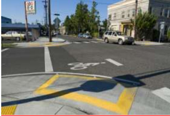
Example of a truck apron, extending the curb making it easier for pedestrians to cross the street, but maintains the turning radius for large trucks which can mount curb. Photo: Michael McKisson.
