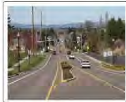
SW 170 th Avenue (south of TV Highway) now includes sidewalks, bike lanes, turn lanes, lighting and landscaping
