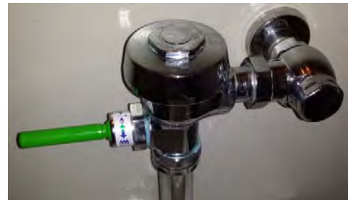
Dual-flush valves at Antoinette Hatfield Hall will help save 420,000 gallons of water a year.
