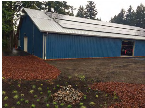
The solar array on the Glendoveer golf cart barn will produce 23,737 kWh of electricity per year.
