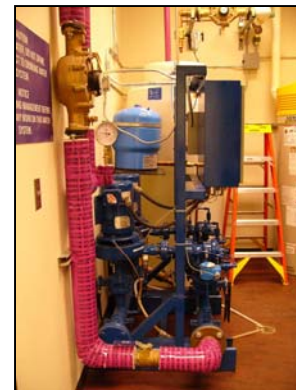
TVWD water reuse system
