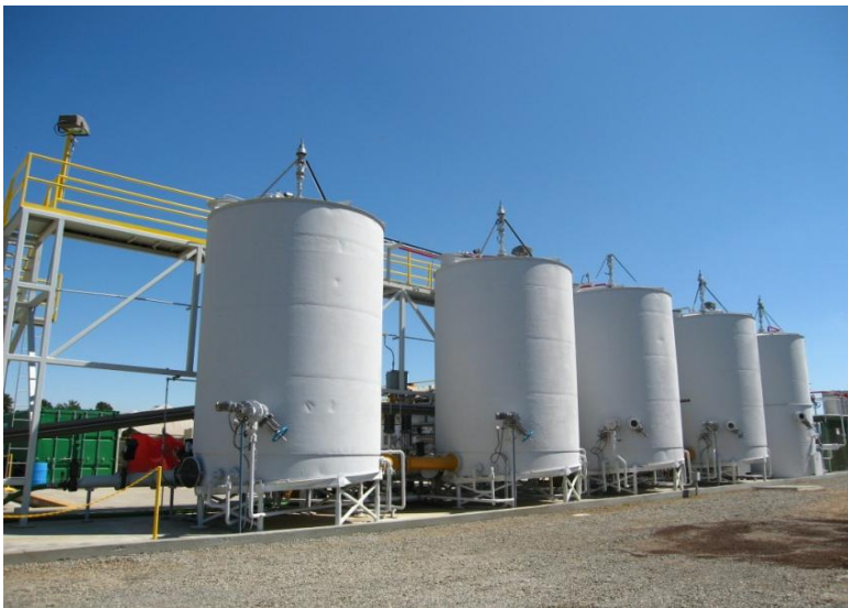
*HDR Photo of Wet system, the University of California Davis Anaerobic Phased Solids (APS) Digester
