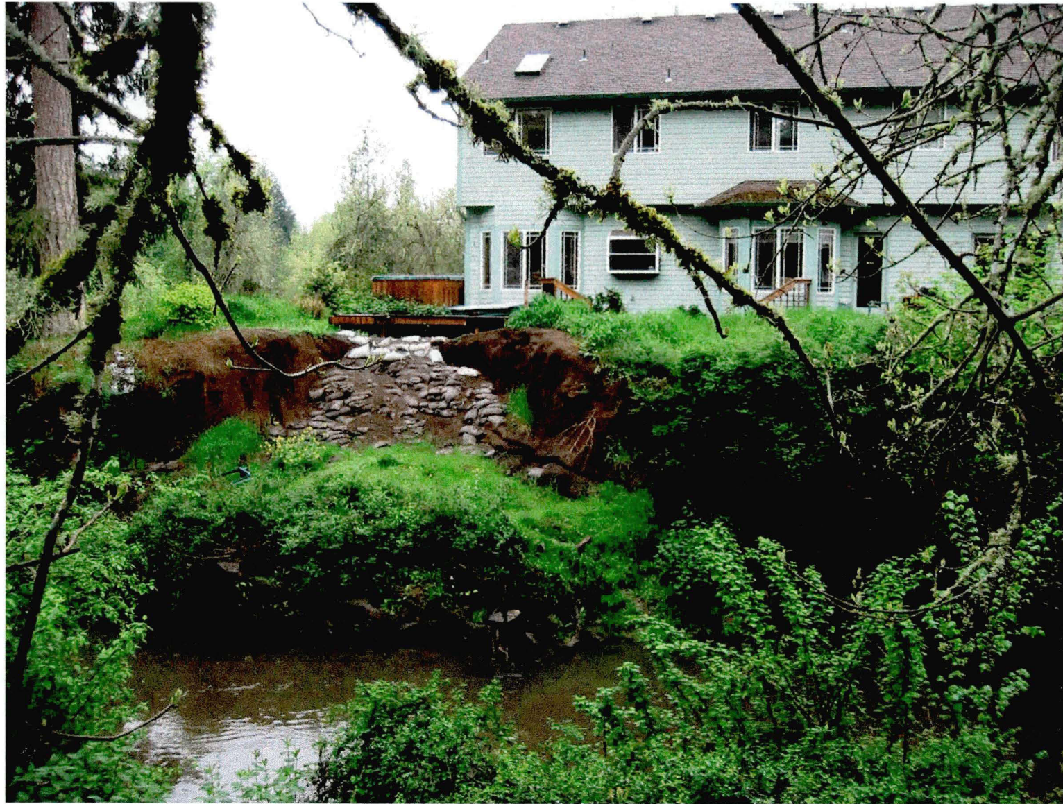
Figure 6: The photograph above was taken from the photo point identified from figure 4 looking west. It shows bank erosion from downstream channel migration along Rock Creek in Hillsboro. The channel eroded the existing riparian buffer and is currently undermining a home built in the 100-year floodplain in 1996. The home is part of the Preston Meadows subdivision permitted in 1995. Current balance cut-and-fill regulations required by Metro would make it much more difficult to construct this home today. However current rules do allow parking lots and active recreation facilities in the floodplain and in the path of migrating channels.
