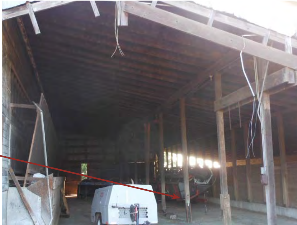
STABILIZE OR REPLACE ACCESSORY #1. CURRENT CONDITION IS POTENTIALLY HAZARDOUS.
