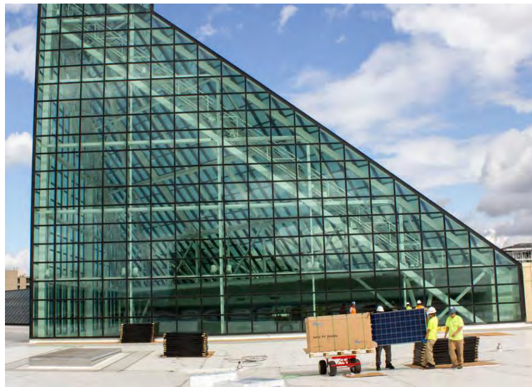
SolarCity began installing 6,500 solar panels at the Oregon Convention Center in September 2015.
