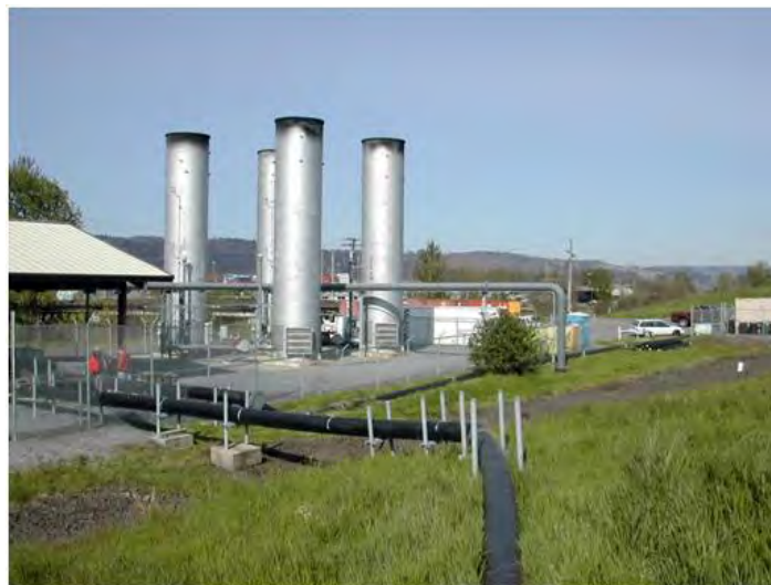
St Johns Landfill Flare Facility
