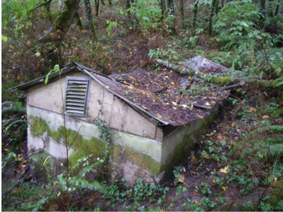
Collapsed springhouse at the top of main stream on north property
