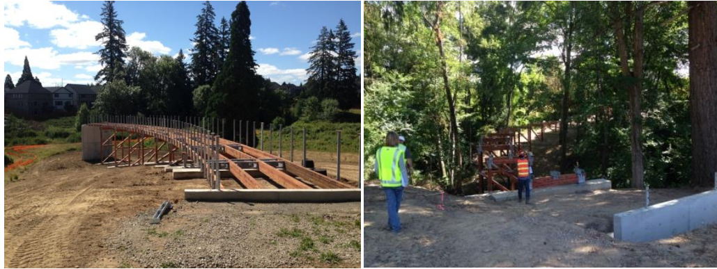
Orenco Woods Nature Park Forest Canopy Bridge and Rock Creek Trail Bridge
