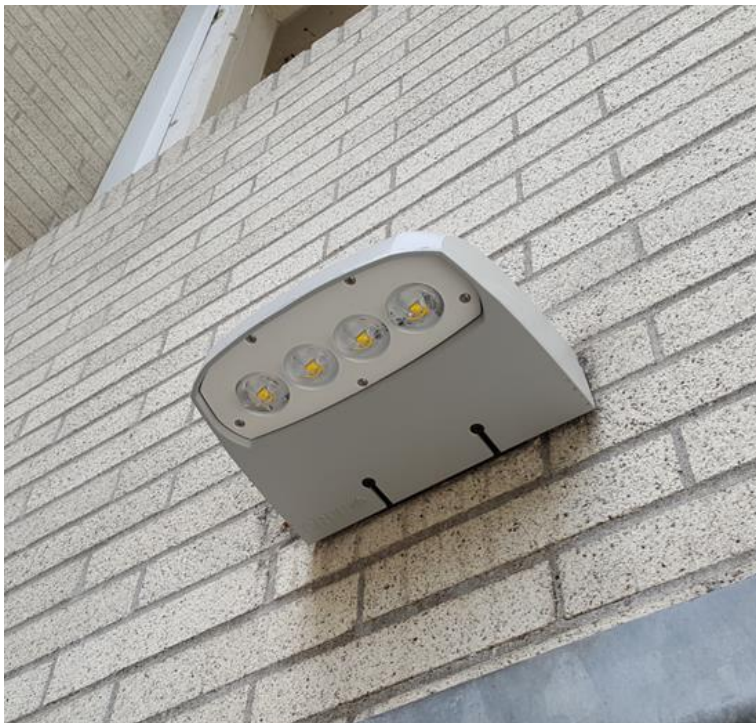
One of the several new LED light fixtures at Metro Regional Center
