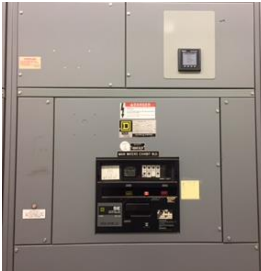
New electrical submeter will monitor energy savings from energy efficiency upgrades at Steller Cove
