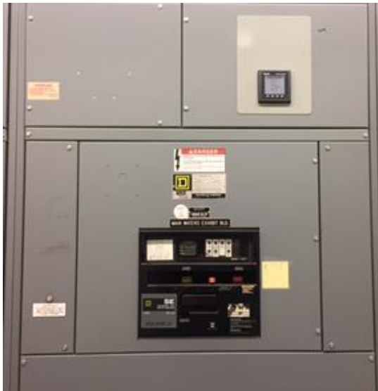
New electrical submeter will monitor energy savings from energy efficiency upgrades at Steller Cove
