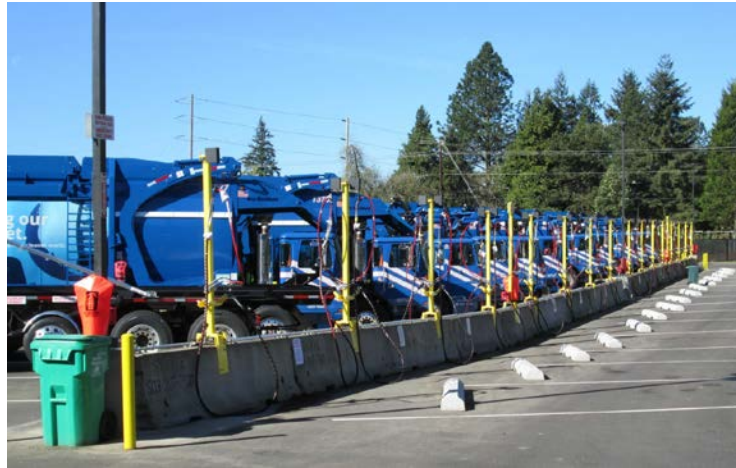
Site of compressed natural gas filling station at WRI.
