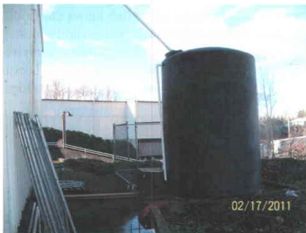
Figure 2 5000 gallon rain water storage tank behind the truck wash
