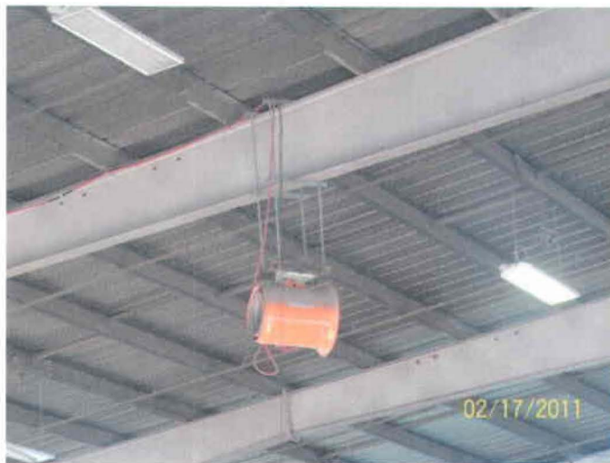
Figure 1 Energy efficient lighting and mister Bay 3
