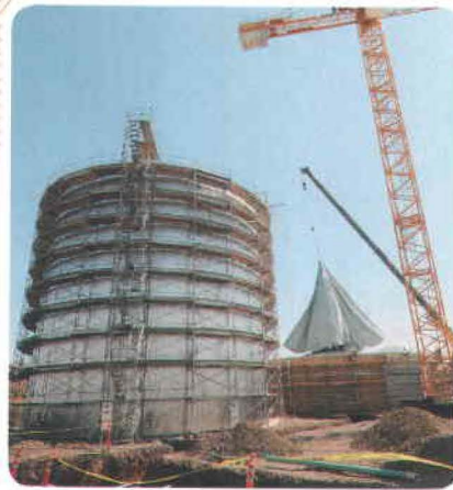
The continuously stirred tank reactor, CSTR, where heated waste digests in an oxygen-free environment, takes shape on left. Smaller crane on right hoists inflatable top for the biogas storage tank.
