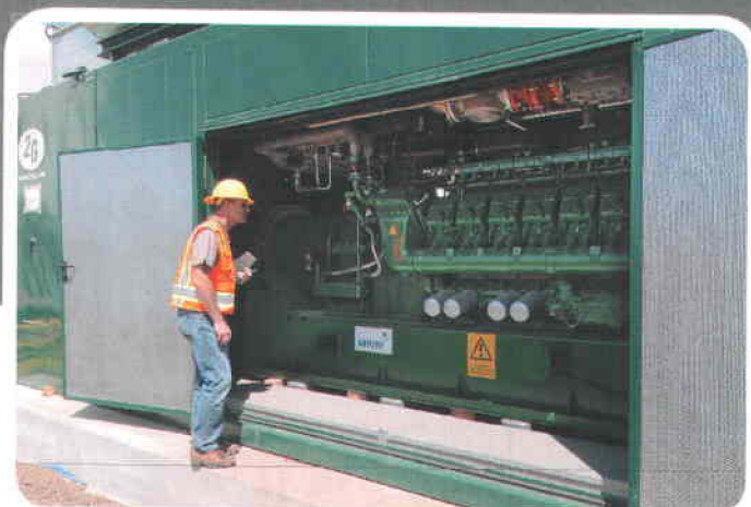
A look at the engine inside the co-generation unit and some of its 16 cylinders. The engine turns a generator to create electricity.
