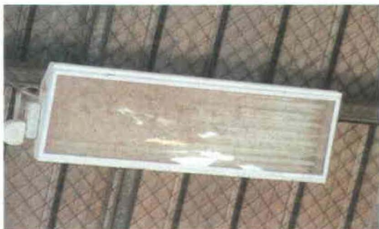
Figure 1 Energy efficient lighting and BMPs ("off").
