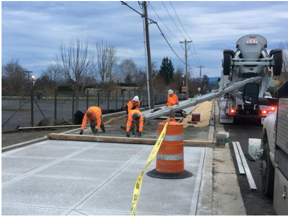
Arata Road sidewalk work near 223 rd Ave Photo courtesy of Multnomah County
