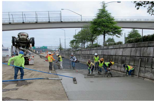
Adding an auxiliary lane on I-205 NB from I-84 EB to Killingsworth, Photo courtesy of ODOT
