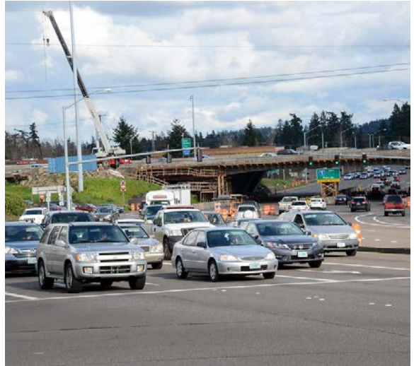
Construction on I-5: North Tigard Interchange (Lower Boones Ferry Road), Photo courtesy of ODOT
