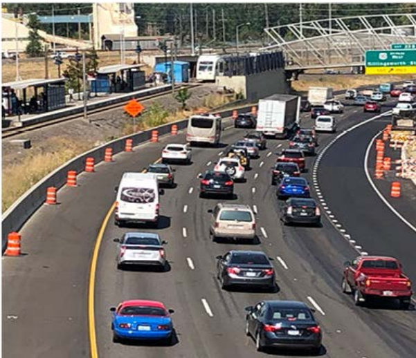
New auxiliary lane on I-205 NB from I-84 EB to Killingsworth, Photo courtesy of ODOT
