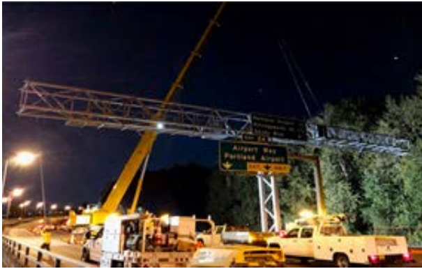
Night work on I-205 Johnson Creek to Glen Jackson Bridge Project, Photo courtesy of ODOT
