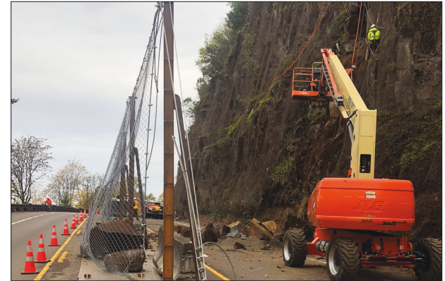
An example of rock scaling work to reduce the risk of rocks falling on a roadway.
