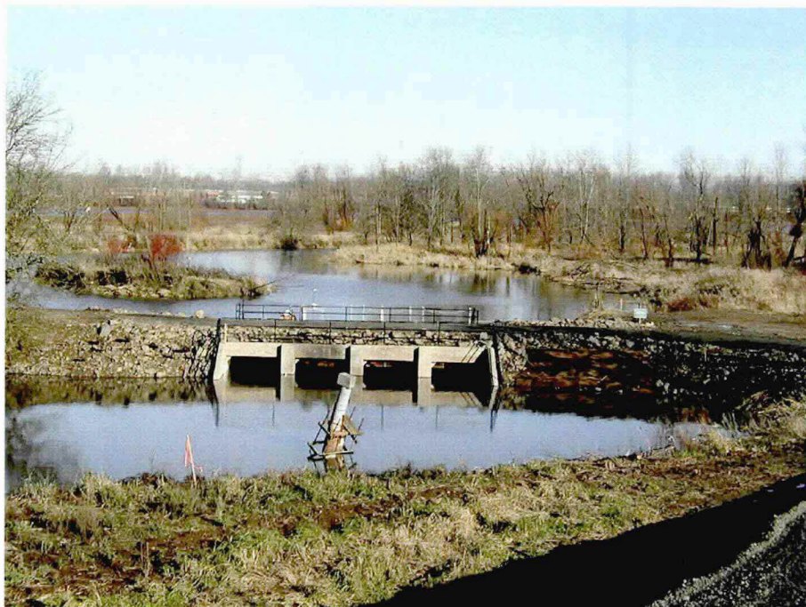
These photographs were taken of the Smith-Bybee earth dam and water control structure in September 2003 and December 2003, respectively.
