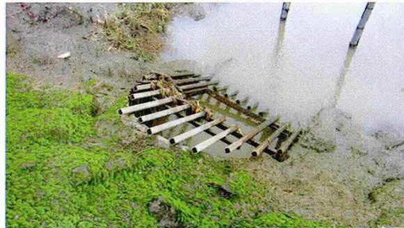
Missing hinged door on NWCS (not immediate need)
