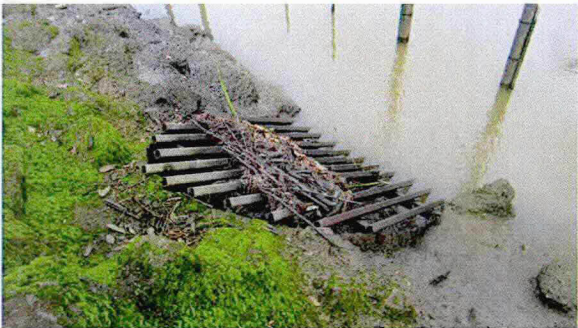
Debris on NWCS trash rack
