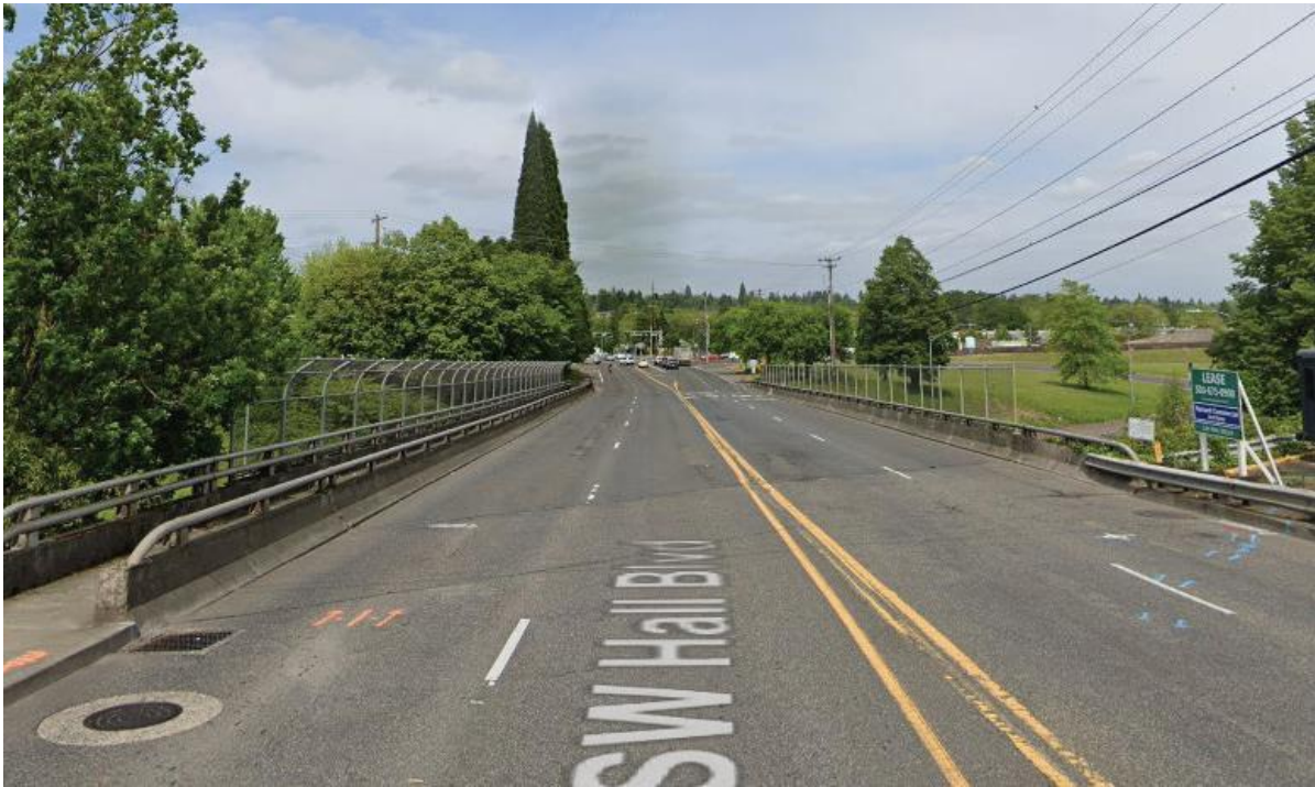
Existing Conditions on Hall Blvd over OR217 (OR217: OR10 – OR99W) Photo Courtesy of ODOT
