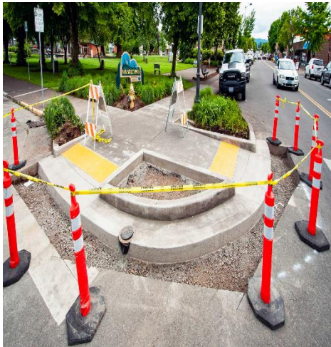
One of many curb ramp projects in the region Photo courtesy of ODOT
