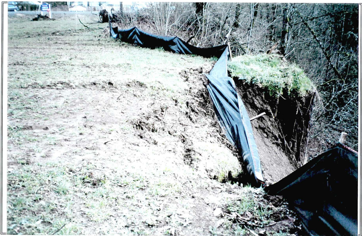
Photo 2. Top of the slide area, note Douglas-fir stump (right side of photo) covered by fill.
