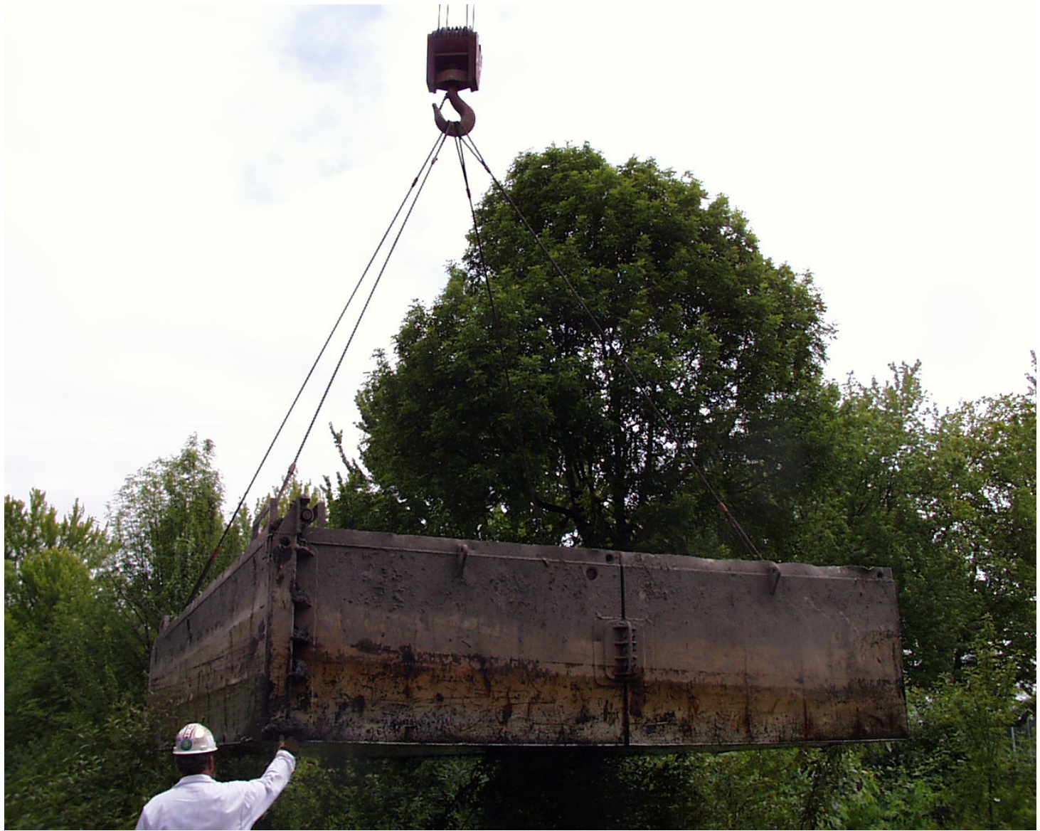
MCDD staff lowering the barge that the the spiderhoe will work off of.
