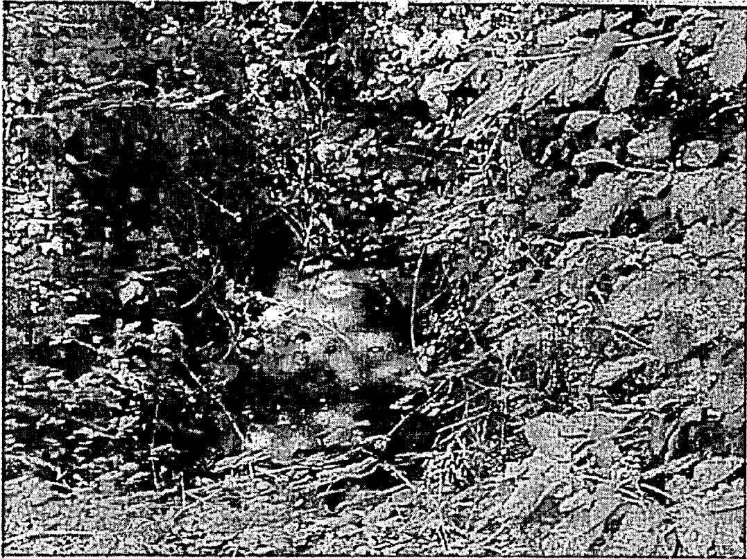
Photo 12. Photo of puddle immediately upstream of Springville Road culvert (upstream view).
