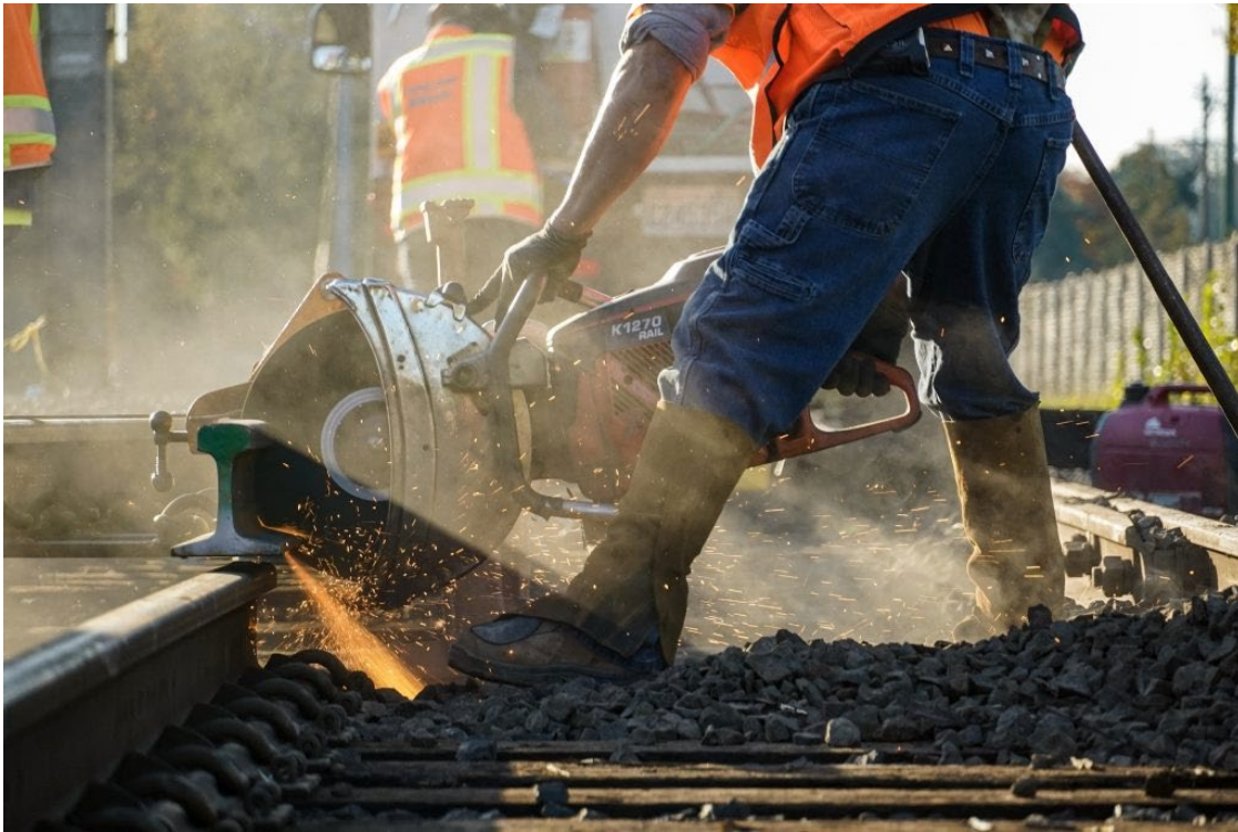
A Better Red MAX Extension and Reliability Project breaking ground one year and four months ago. Photo courtesy of TriMet
