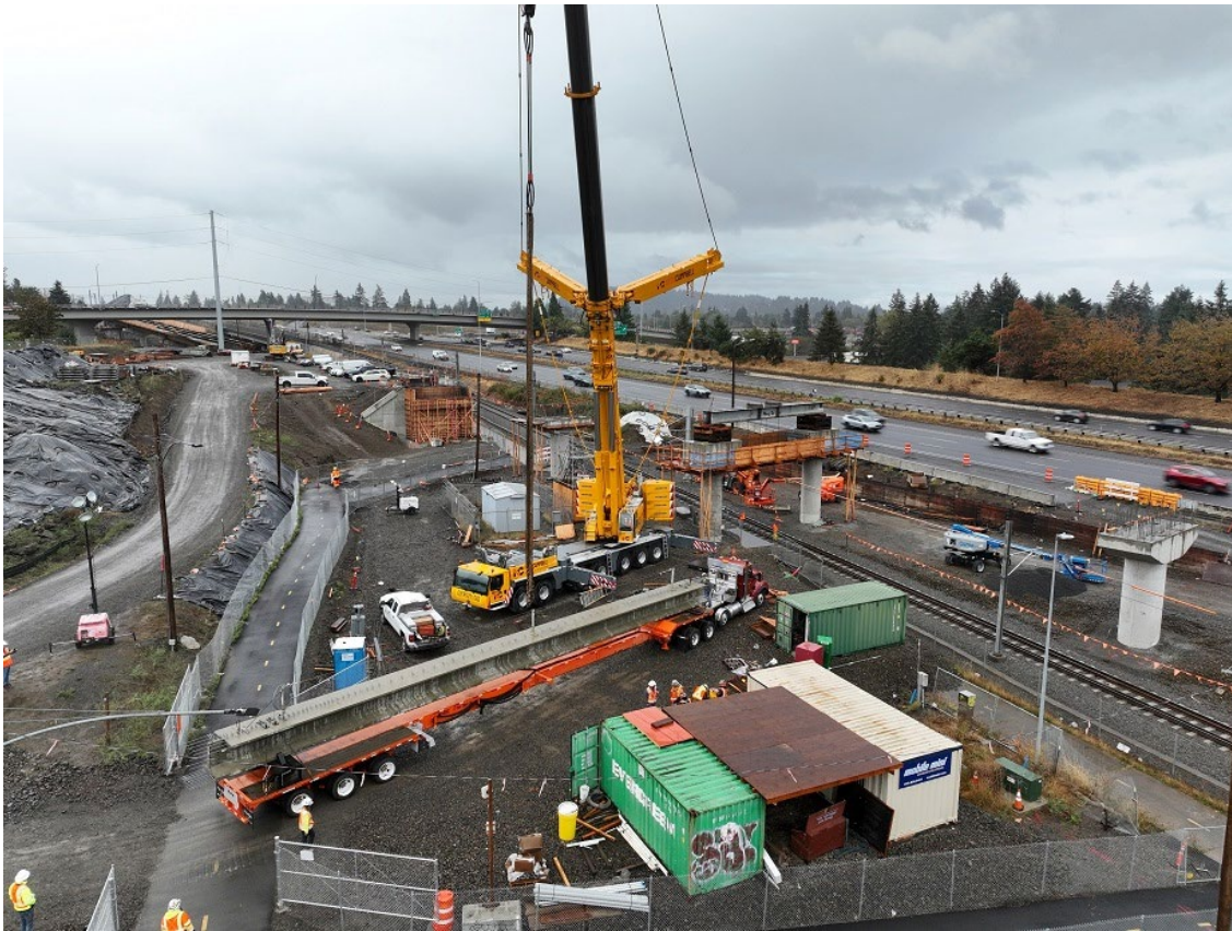
Construction on a section of the MAX Red Line project north of the Gateway Transit Center Photo courtesy of TriMet
