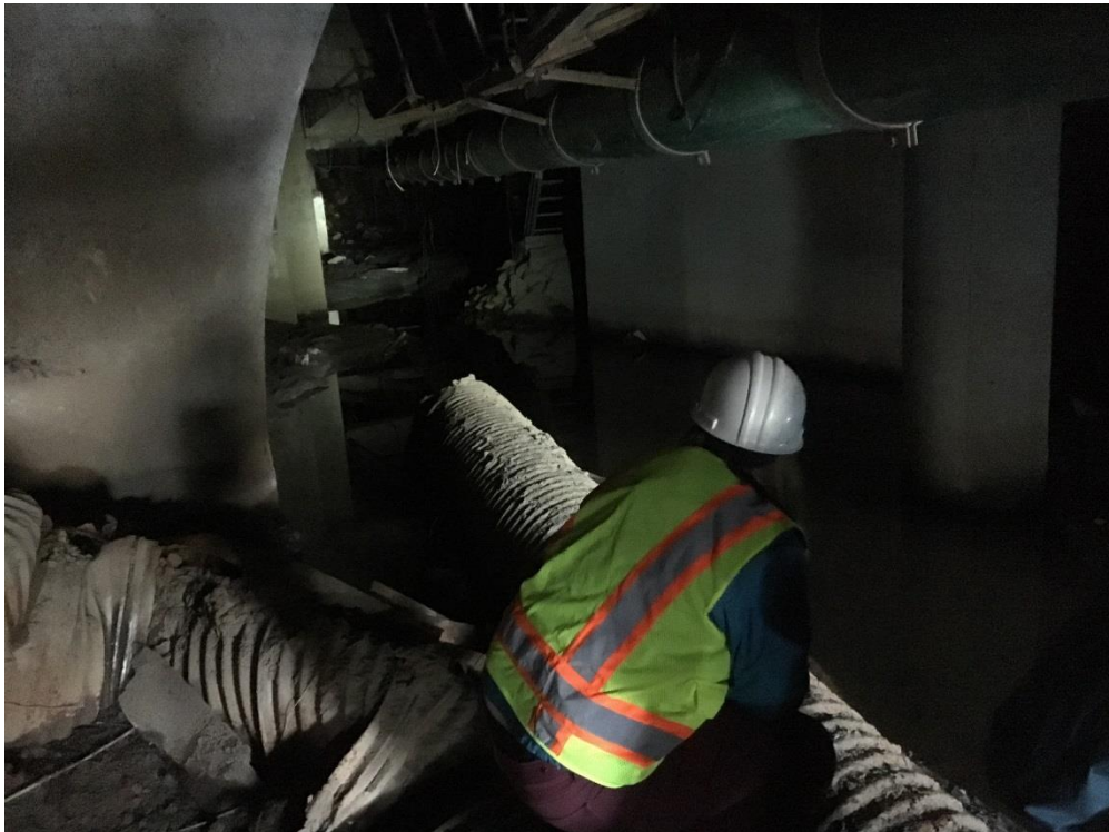
Figure A-4. Photographic views of basalt rock debris and fill material located near the tailrace channel beneath the Boiler Plant.
