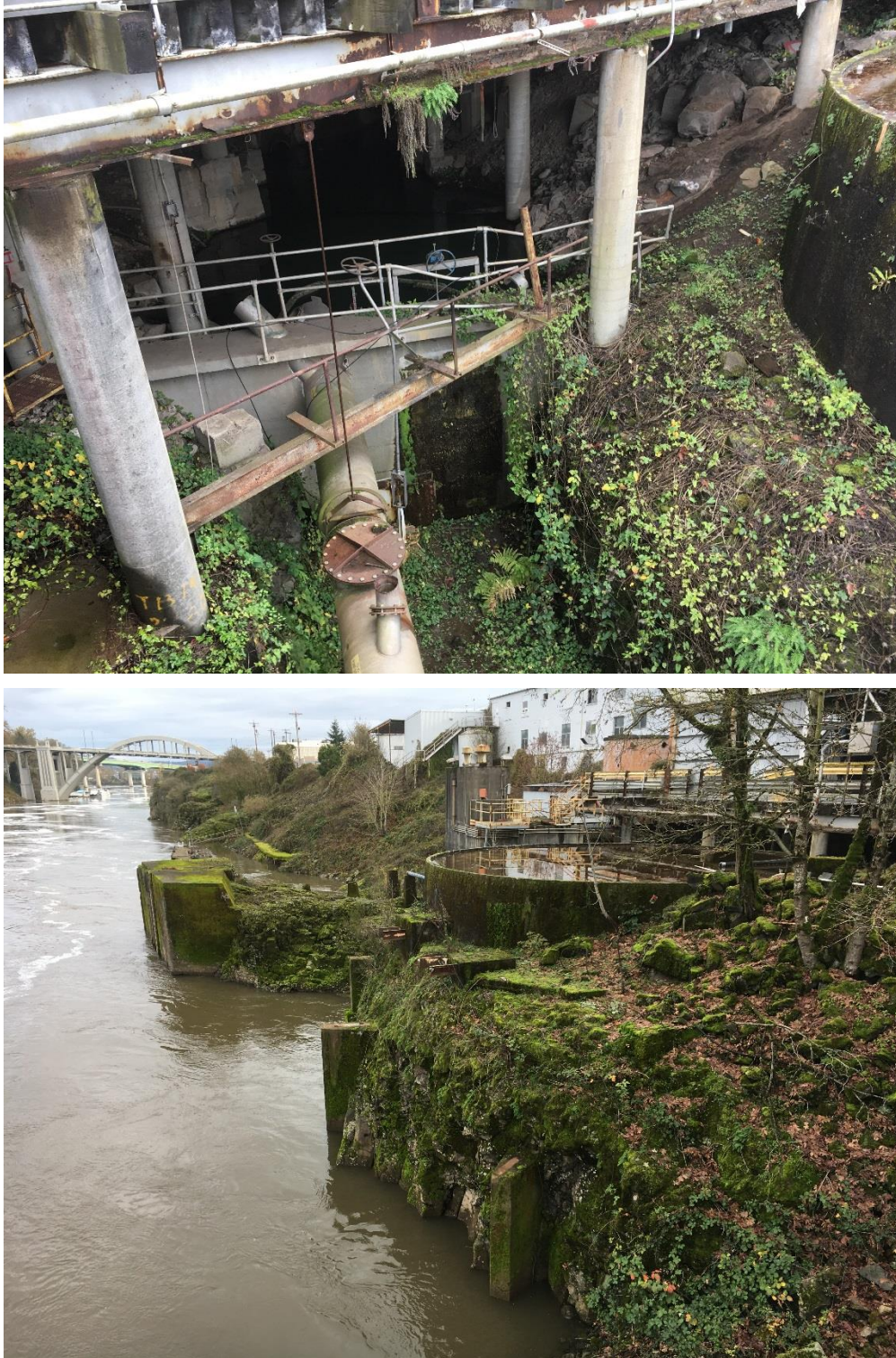
Figure A-3. Photographic views of basalt outcrops and rock debris located near the millrace outlet beneath No. 3 Paper Machine Building #2 (top) and the Circular Tank Foundation 1 (bottom).
