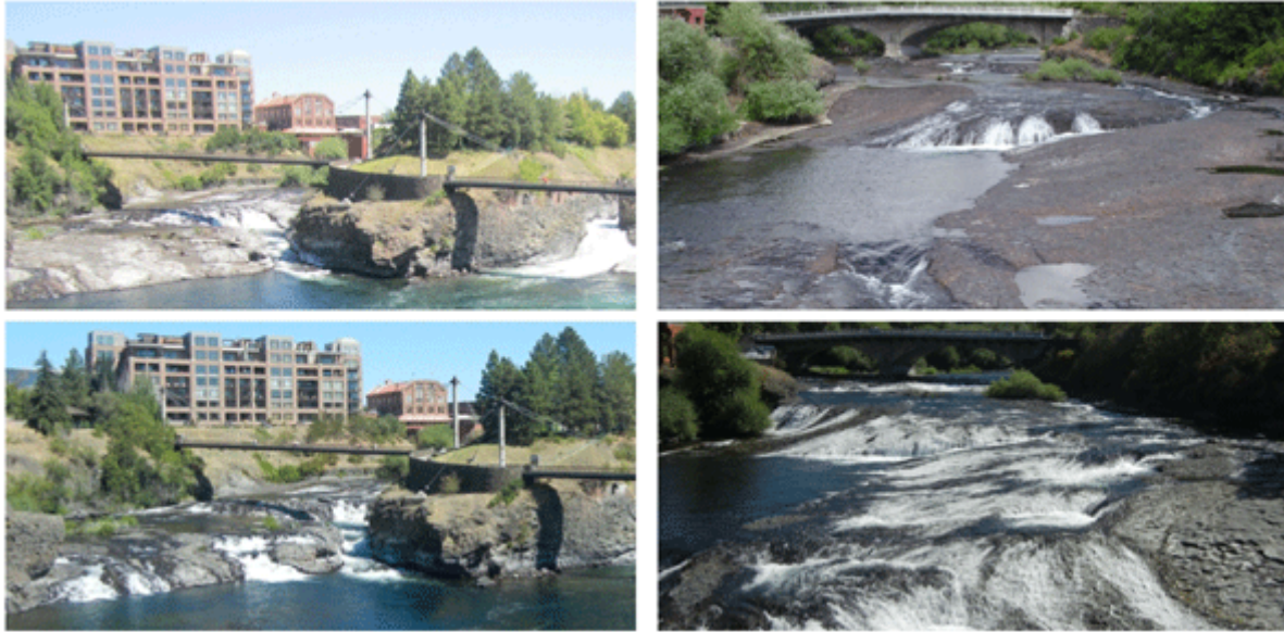
Figure 3, North channel before (top at 500cfs) and after (bottom at 300cfs) construction.
