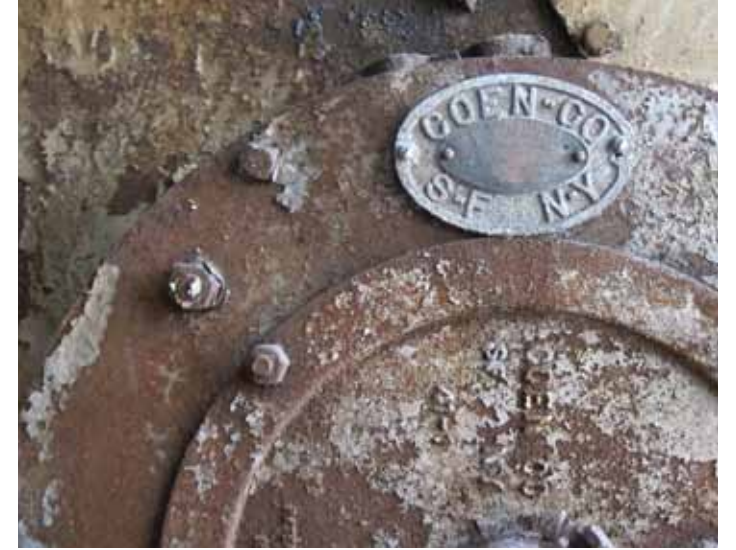
Mill G Boilers
